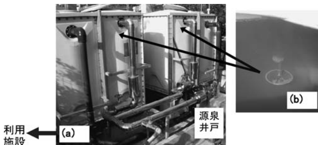
Fig. 5 Separation and removal equipment for methane gas using water tanks combined with sprinkling device.
